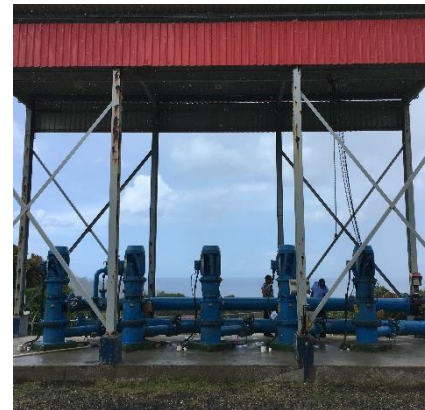
THEOBALD WTP PUMPING STATION, 2019
